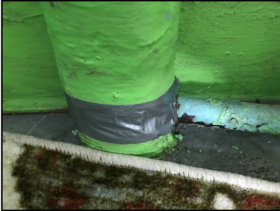
Photo 3: Asbestos containing TSI in restroom 2 on heat piping
