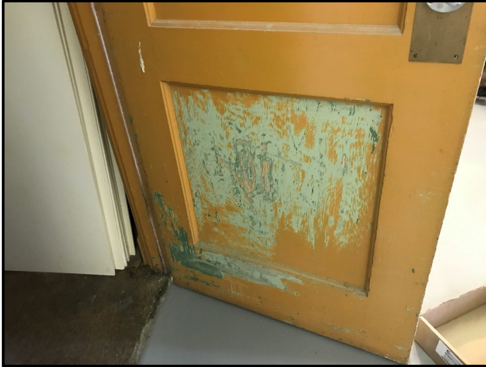
Photo 5: PCB containing paint was found on the interior and exterior of the janitor closet door. Assume all doors are PCB containing.
