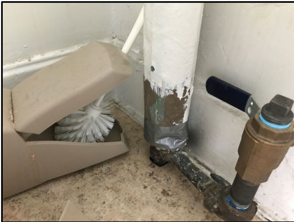
Photo 4: Asbestos containing TSI in restroom 1 on heat piping
