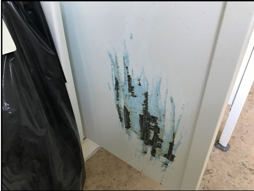
Photo 6: PCB containing paint found on the divider stalls in restroom 2. Assume at restroom dividers are PCB containing.
