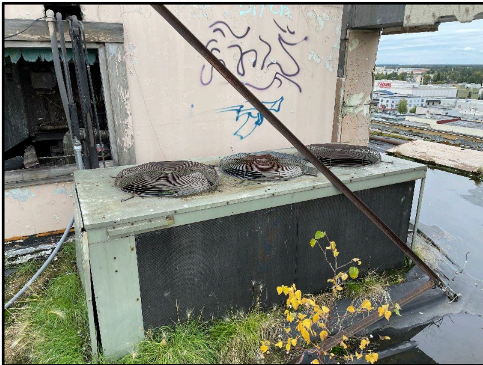
Photo 24: Air handling condenser (R-25) - Roof
