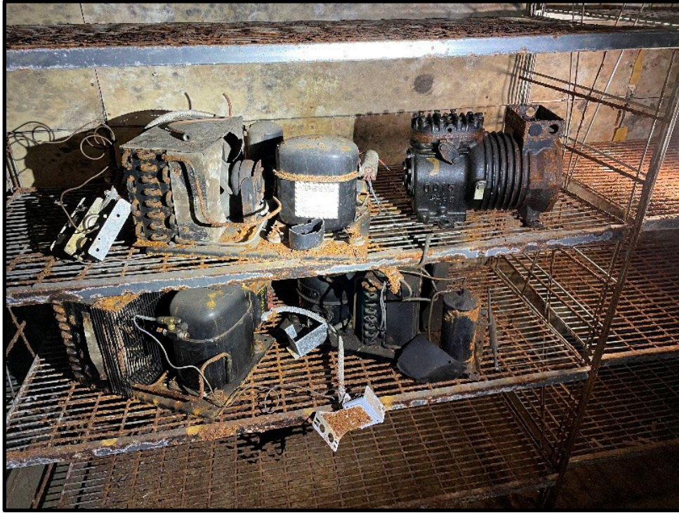
Photo 1: Refrigeration / air conditioner parts (R-1) - Basement
