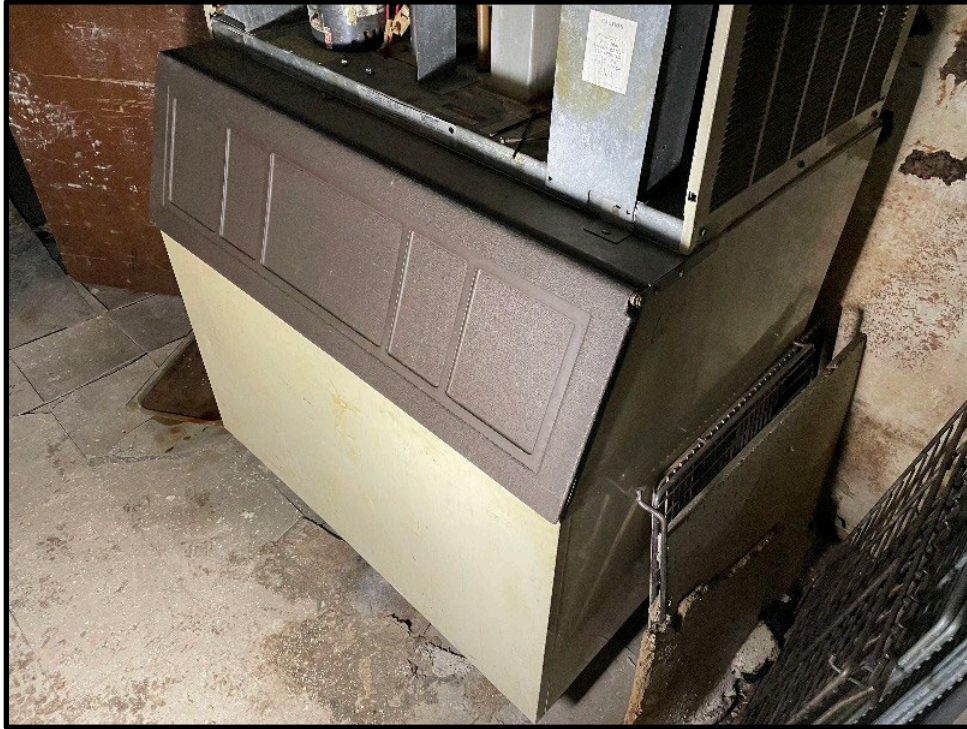
Photo 7: Ice machine (R-9) – Ground floor
