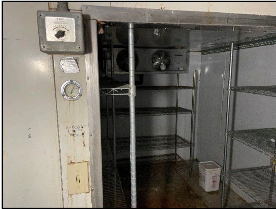
Photo 13: Walk-in freezer inside (R-14) – Penthouse floor
