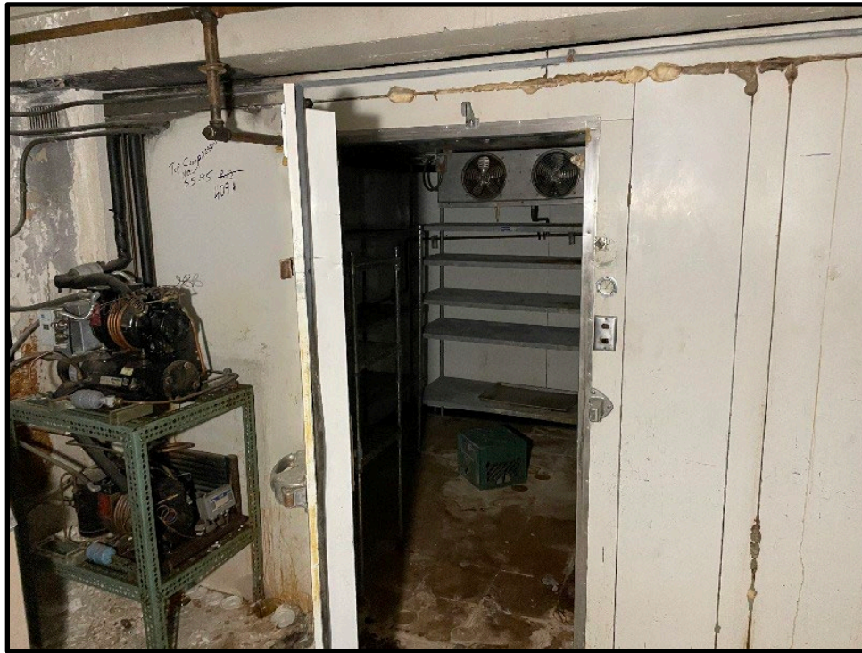
Photo 11: Walk-in refrigerator inside (R-13) – Penthouse floor
