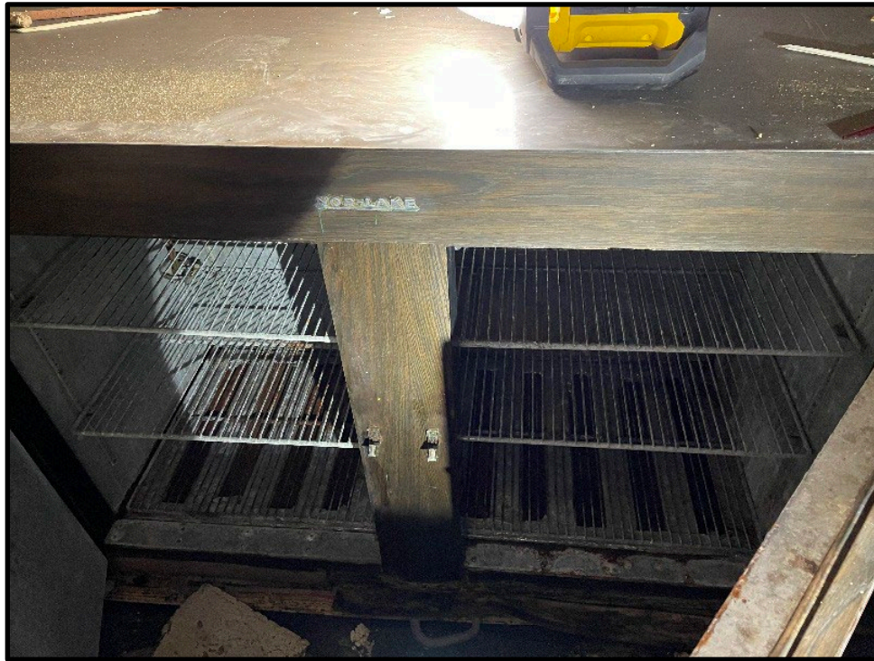
Photo 3: Typical under cabinet refrigerator (R-2) – Ground floor
