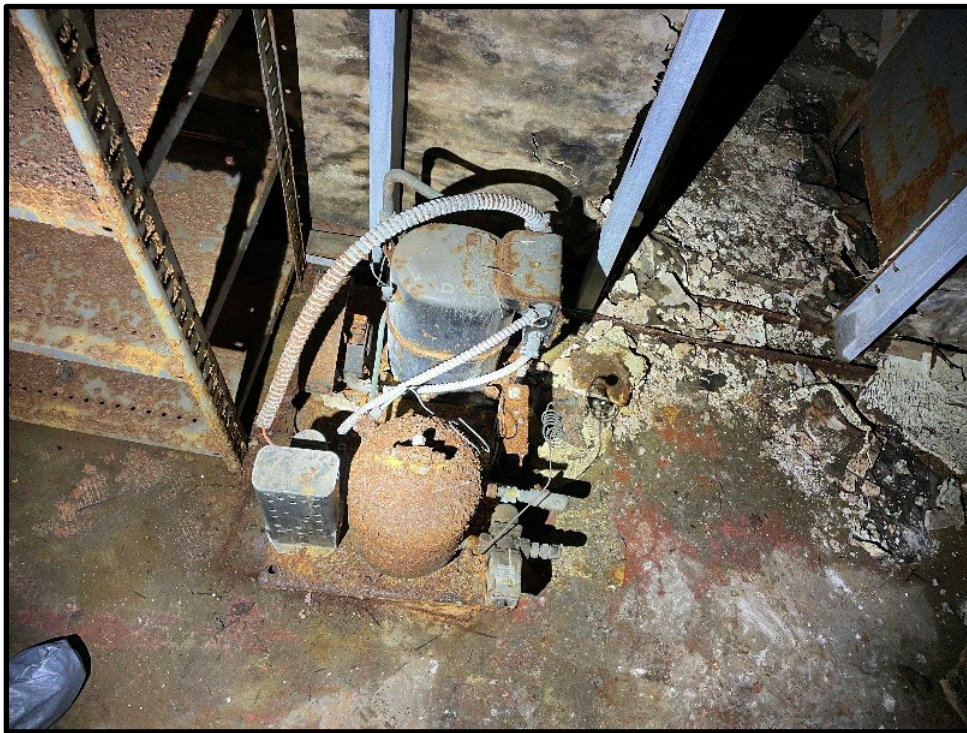
Photo 2: Refrigeration / air conditioner parts (R-1) - Basement
