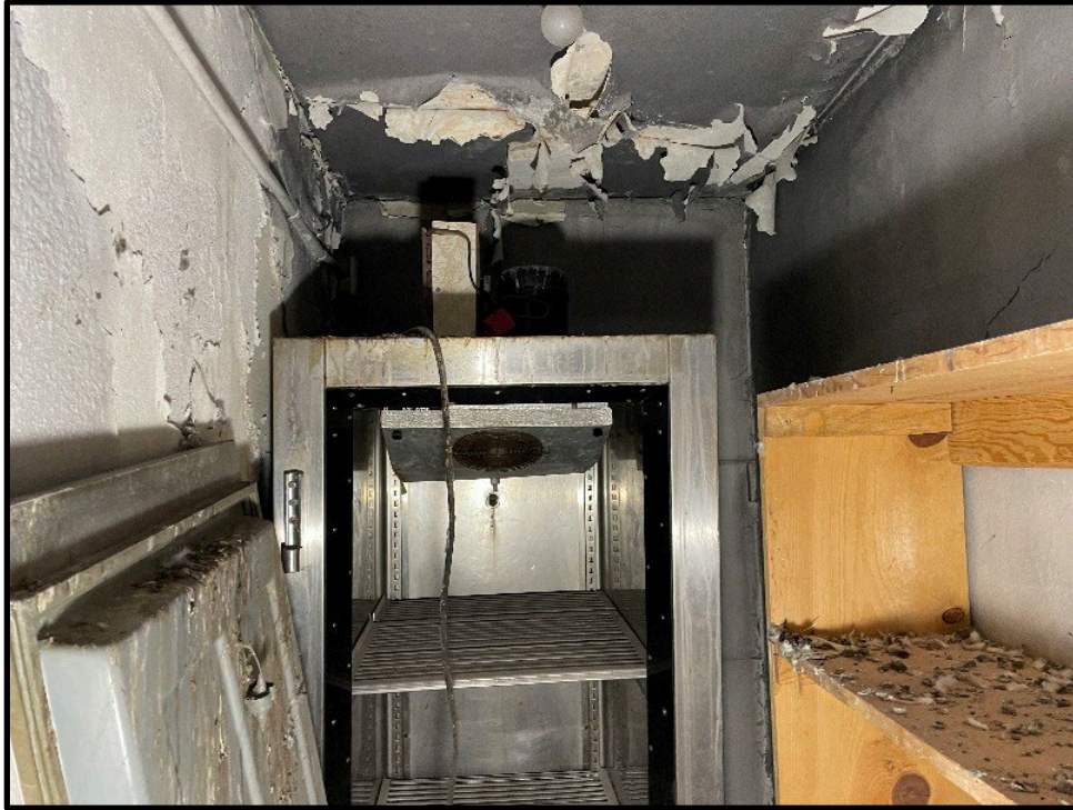
Photo 17: Standup refrigerator (top) (R-19) – Penthouse floor
