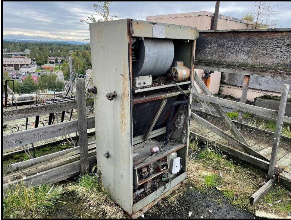
Photo 23: Air handling unit (R-24) - Roof
