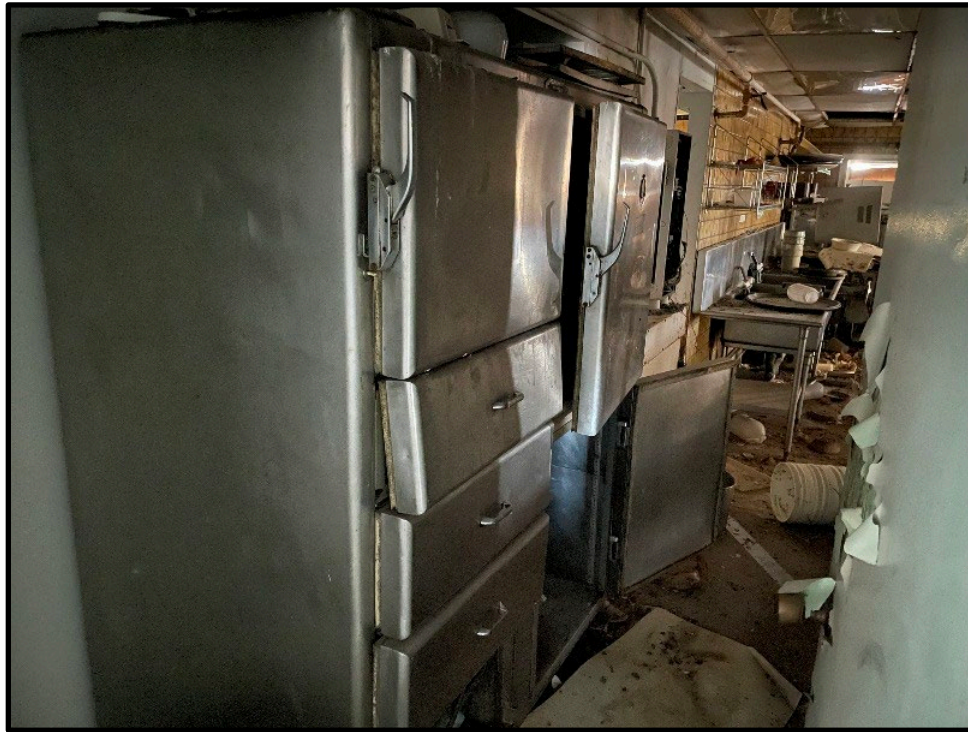
Photo 19: Double standup refrigerator (R-20) – Penthouse floor
