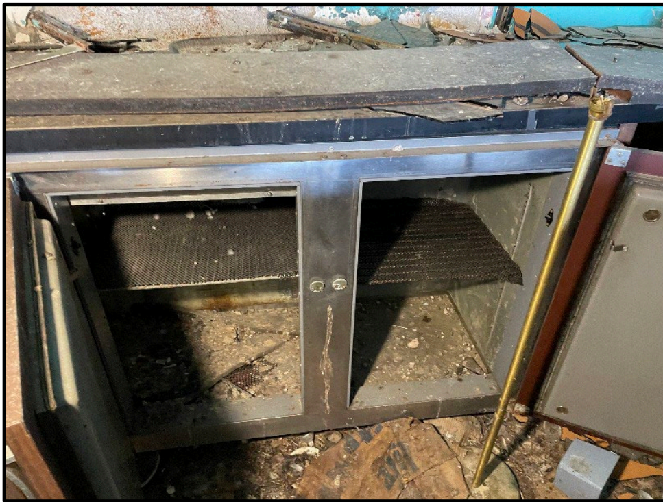
Photo 16: Under cabinet refrigerator (R-18) – Penthouse floor
