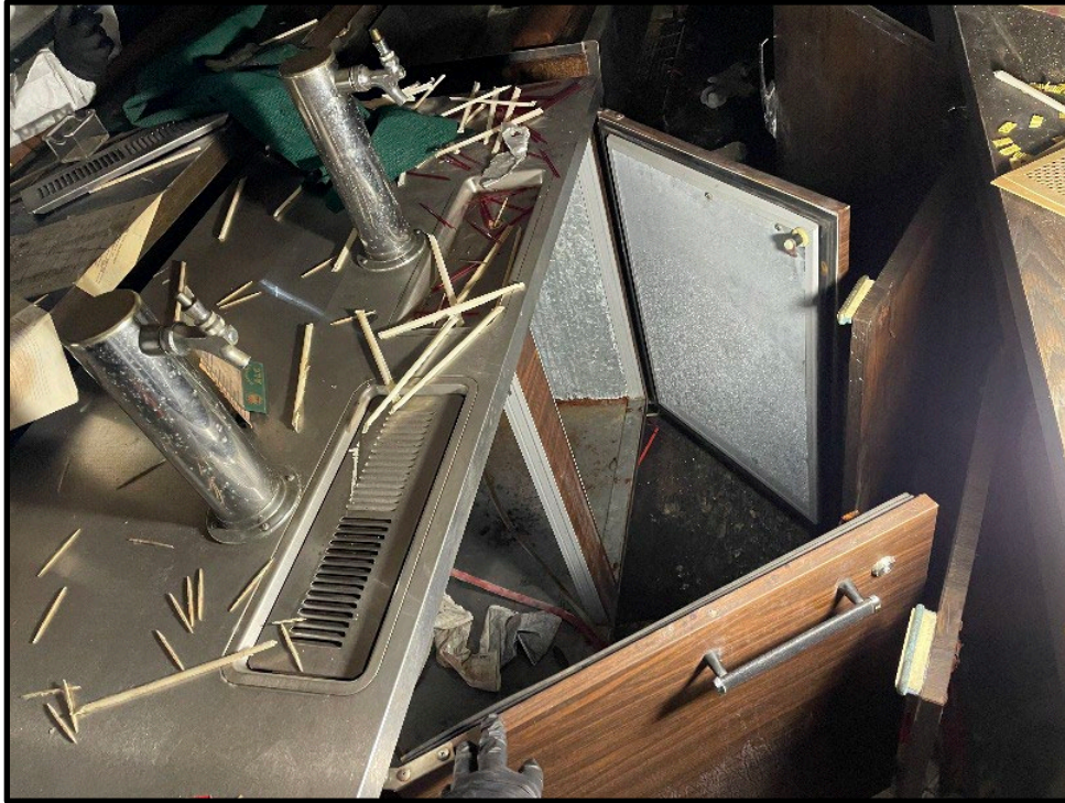
Photo 5: Keg refrigerator (R-3) – Ground floor
