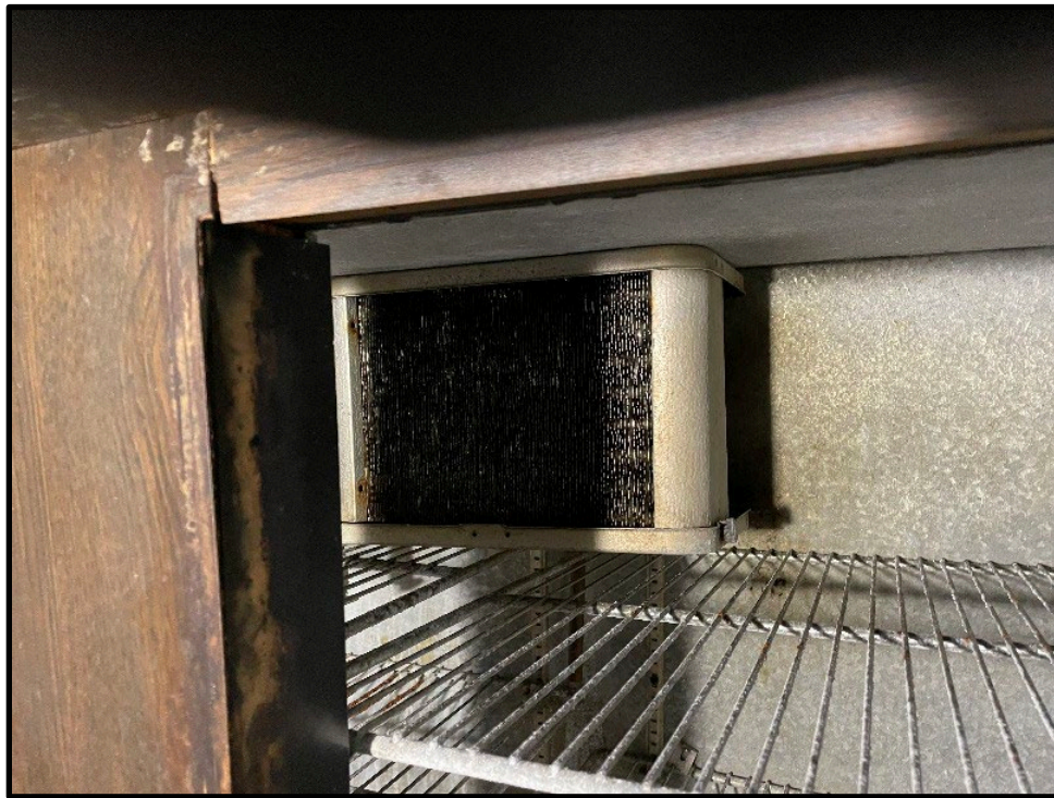
Photo 4: Typical under cabinet refrigerator close-up (R-2) – Ground floor
