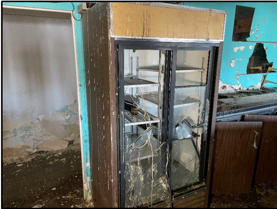
Photo 15: Glass display refrigerator (R-17) – Penthouse floor
