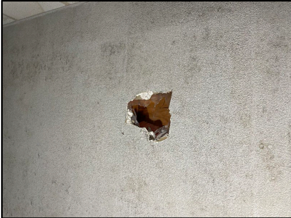
Photo 4: Main Floor – PCB Sample M2 collected from off-white textured paint near entryway.
