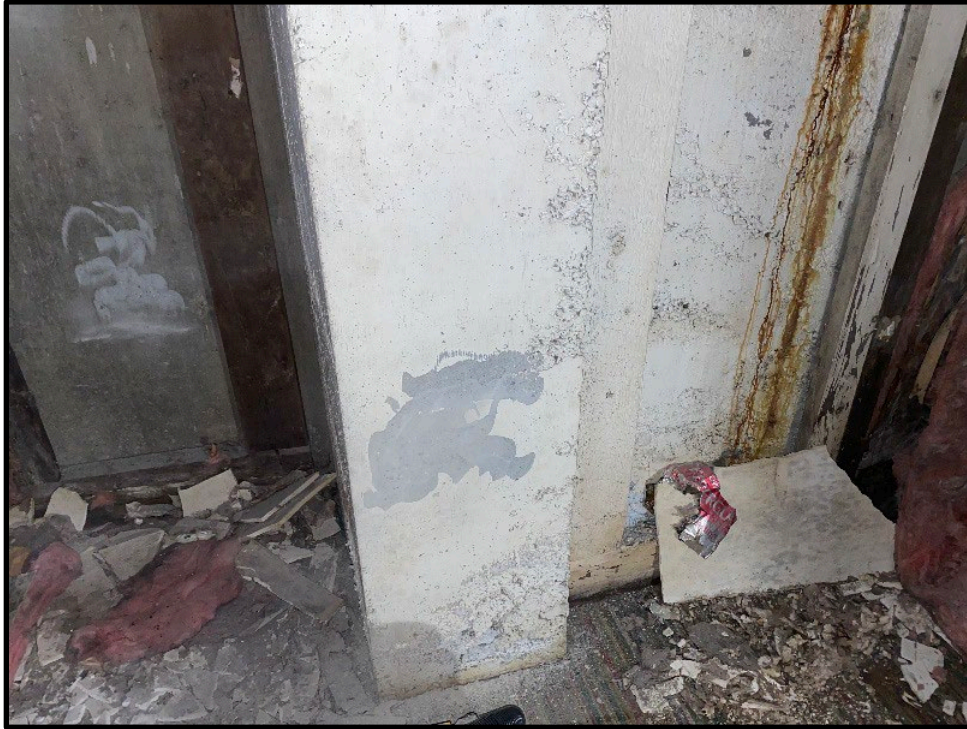
Photo 1: Basement – PCB Samples B1 & B2. Sample B1 collected from unpainted concrete in left of photo. Sample B2 collected from white painted concrete column in center.
