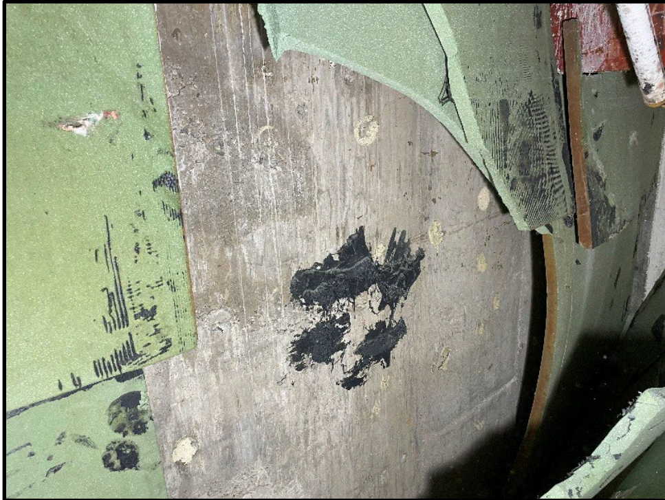
Photo 2: Basement – Stairwell exterior wall showing white and red painted stairs/supports in upper right of photo. Black mastic contains asbestos.
