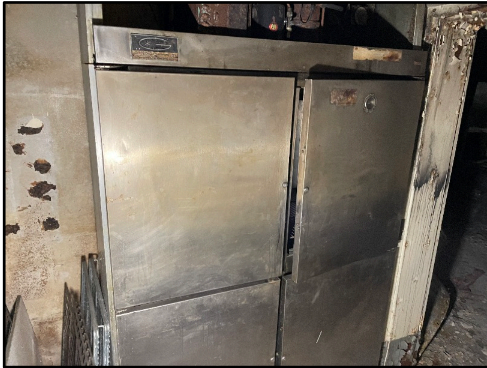
Photo 9: Standup refrigerator (R-7) – Ground floor
