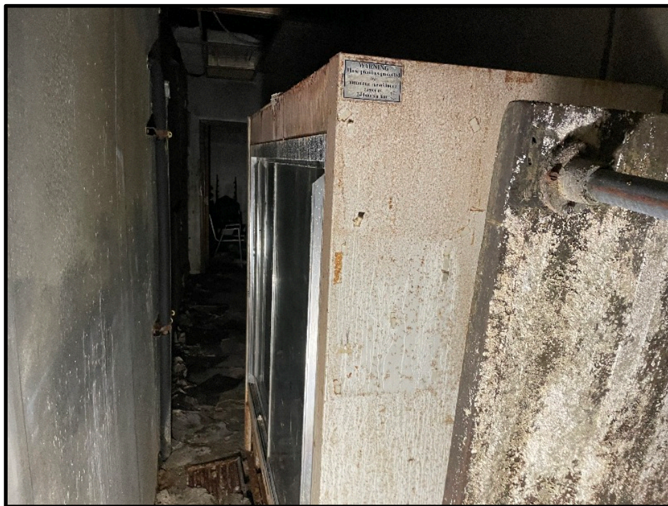
Photo 10: Glass display refrigerator (R-8) – Ground floor
