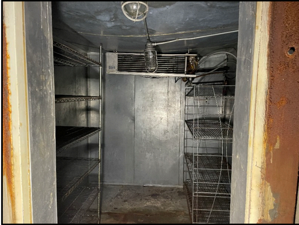
Photo 7: Walk-in freezer (R-5) – Ground floor
