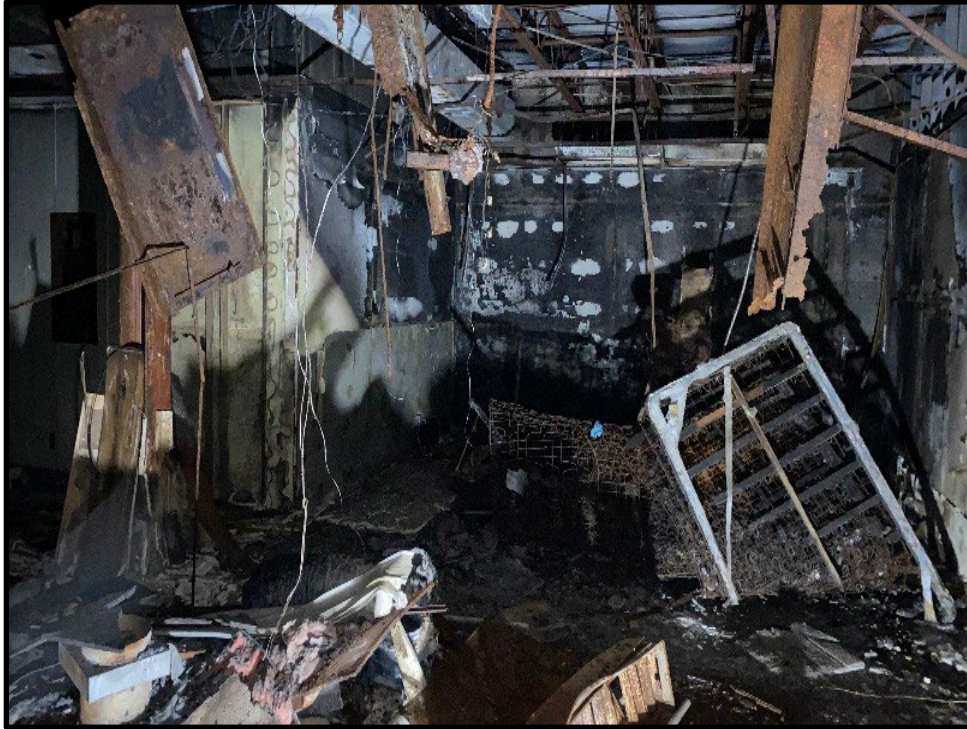
Photo 3: Main Floor – Dining/Conference room fire damage. Black in image is soot and burned materials.
