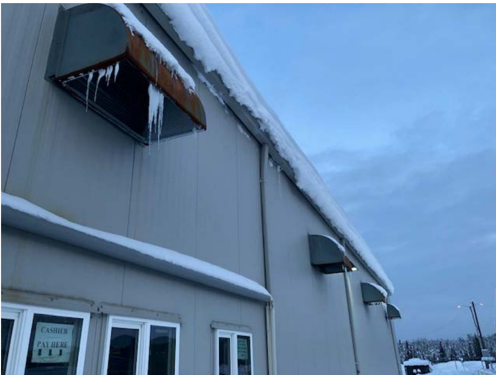
Gutter that needs the heat trace system.
