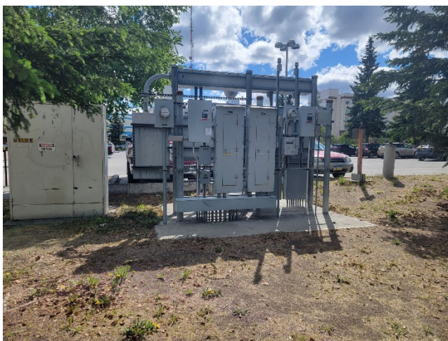
Power Supply to Clock Tower
