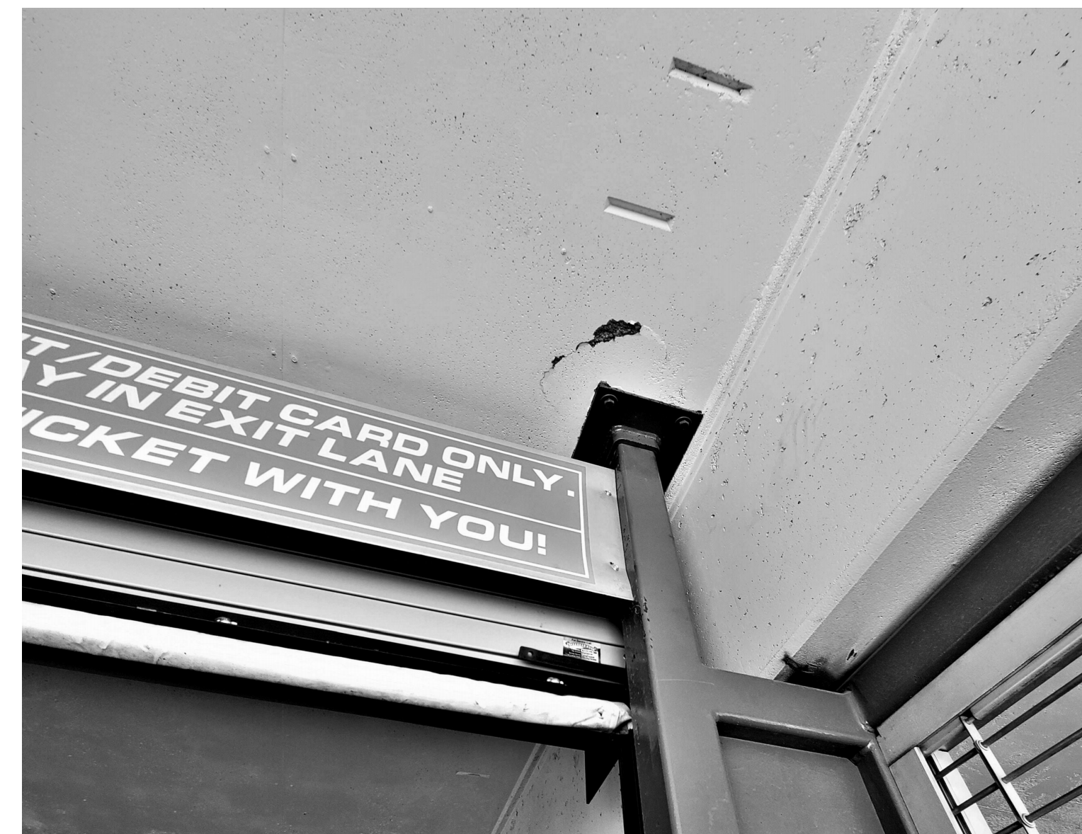
7 REPAIR 7 - SPALLING AT HSS ANCHOR S201 1" = 1'-0"
