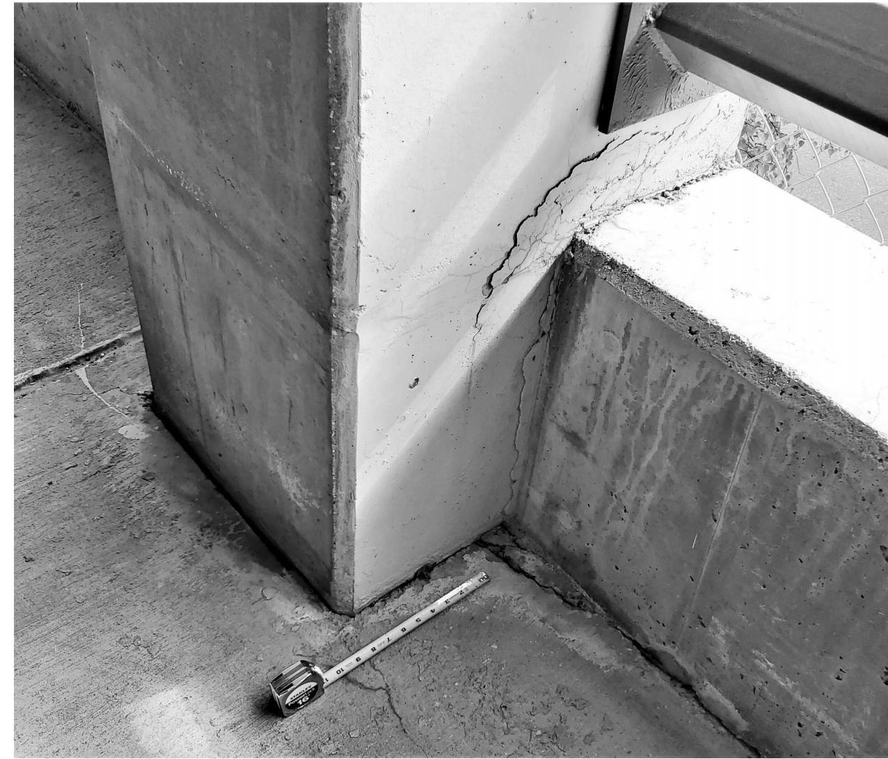
1.A REPAIR 1 - SPANDREL BEAM CRACKING (ABOVE) S201 1" = 1'-0"
