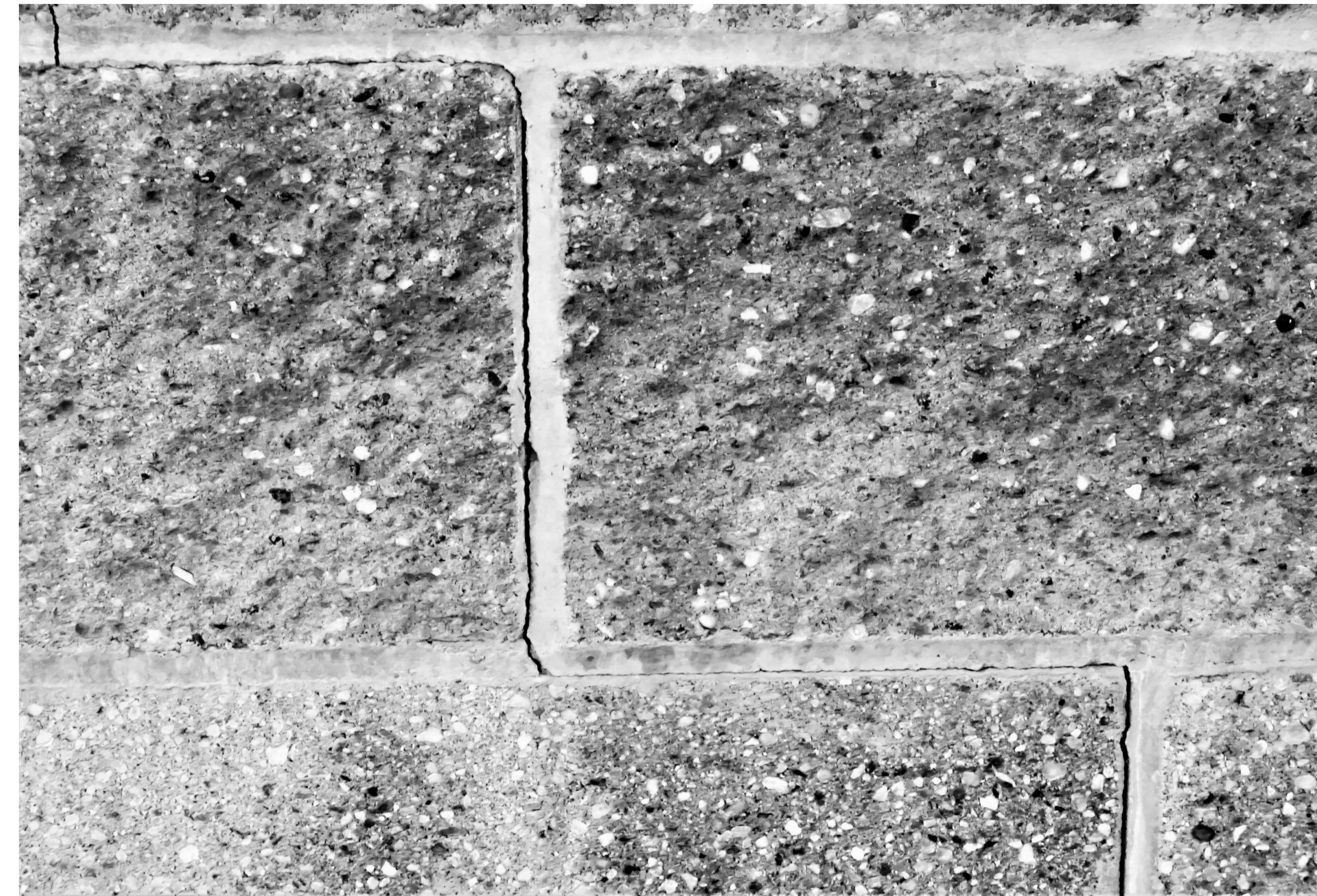
A2 S202 ALTERNATE #2 - REPAIR A2 - CRACKED MORTAR JOINTS AT EXTERIOR CMU FACE 1" = 1'-0"
