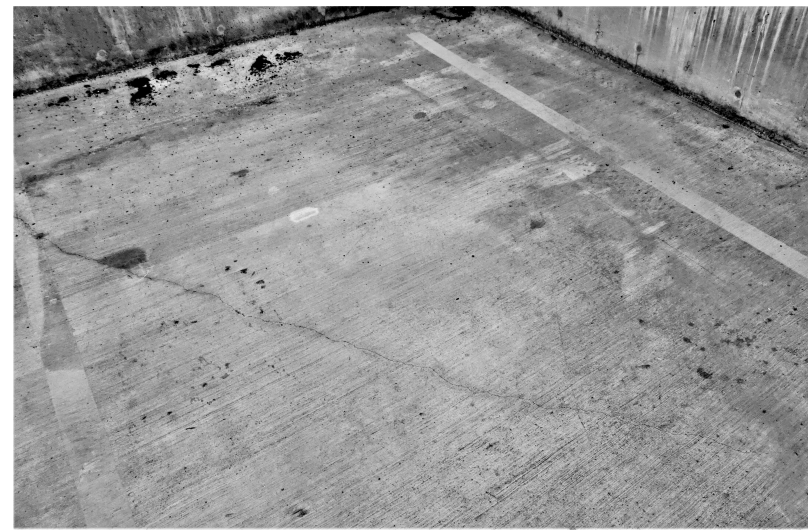
3.B REPAIR 3 - POST TENSION SLAB CRACKING (TOP) S201 1" = 1'-0"
