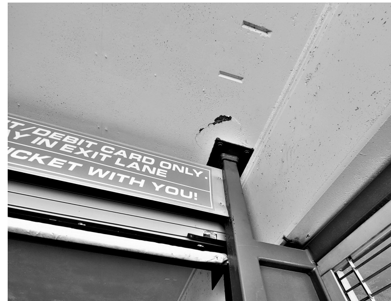
7 REPAIR 7 - SPALLING AT HSS ANCHOR S201 1" = 1'-0"
