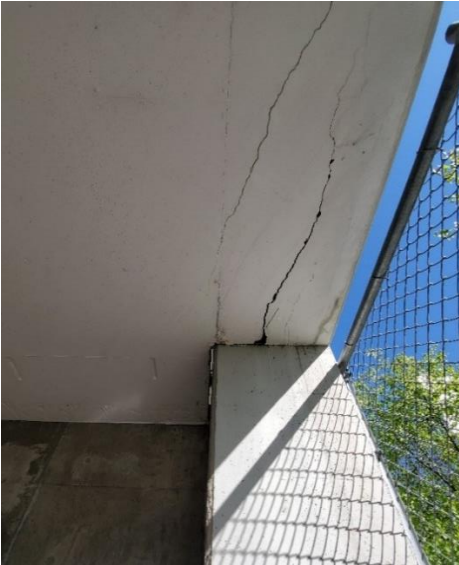
Figure 4: Slab & Spandrel Cracking from Below
