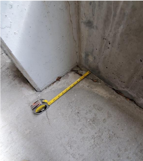
Figure 5: Slab & Spandrel Cracking from Above
