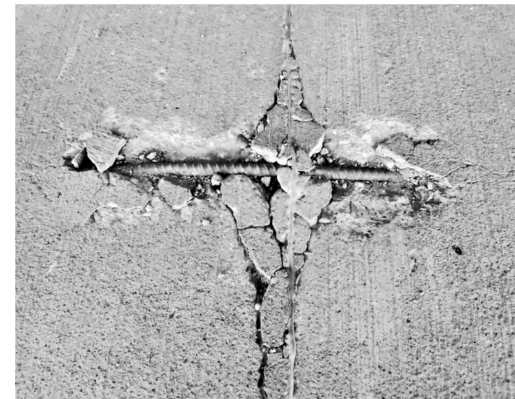
8 REPAIR 8 - DIAMOND SPALLING OF SLAB S201 1" = 1'-0"
