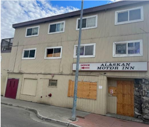
Figure 14. Many vacant buildings need repairs or upgrades.
