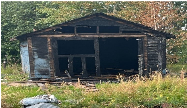
Figure 19: A burned out garage along 9 th Avenue
