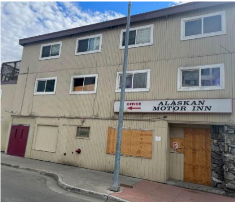
Figure 14. Many vacant buildings need repairs or upgrades.
