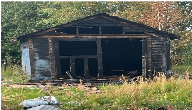
Figure 20: A burned out garage along 9 th Avenue
